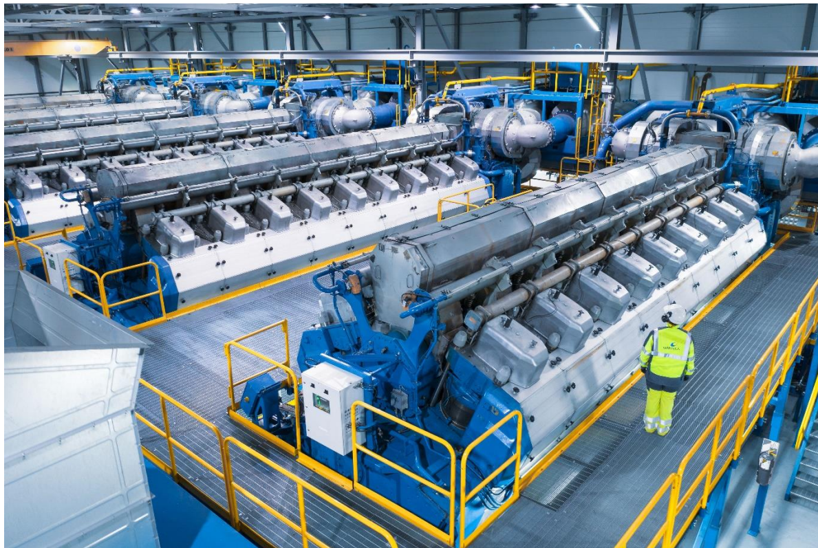
WÄRTSILÄ POWER PLANT FROM THE INSIDE
